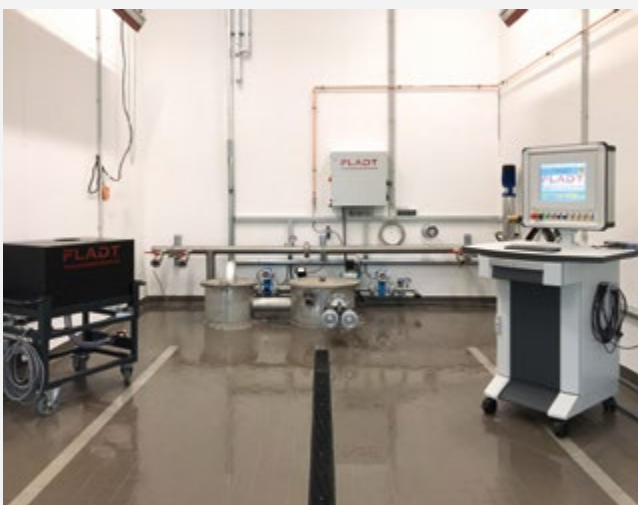
Pump test hall from the inside with ideal connection possibilities for suction and pressure hoses
